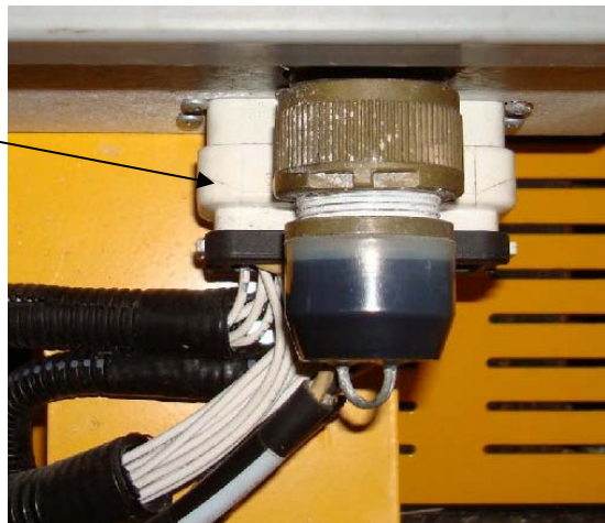
Figure 8-2. Ground Control Panel Receptacle
